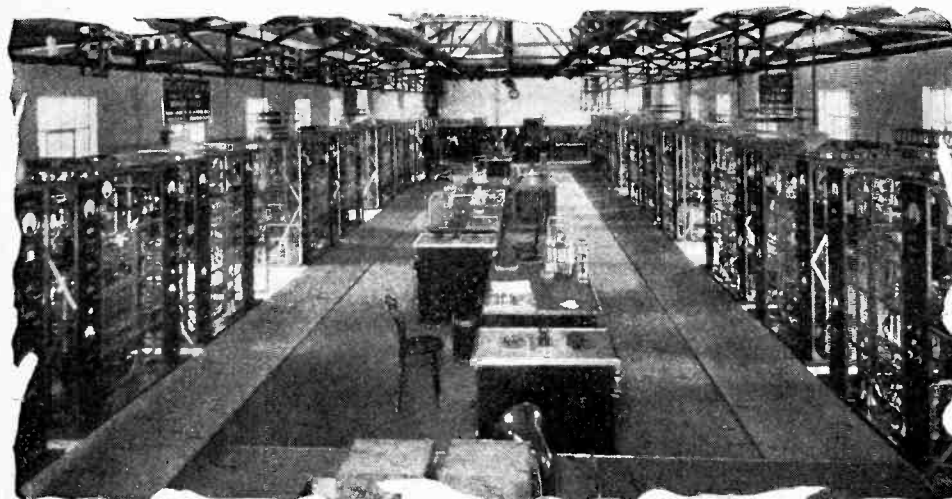
No fewer than eight Marconi beam transmitters are housed in this hall, from which direct communication is maintained with U.S.A., South America, Egypt, Japan and the Far East.
